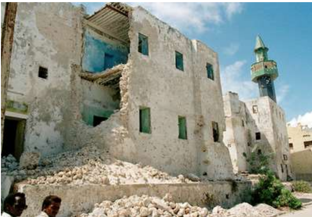
An Image showing a damaged building from Somalian War (1993-1994)
